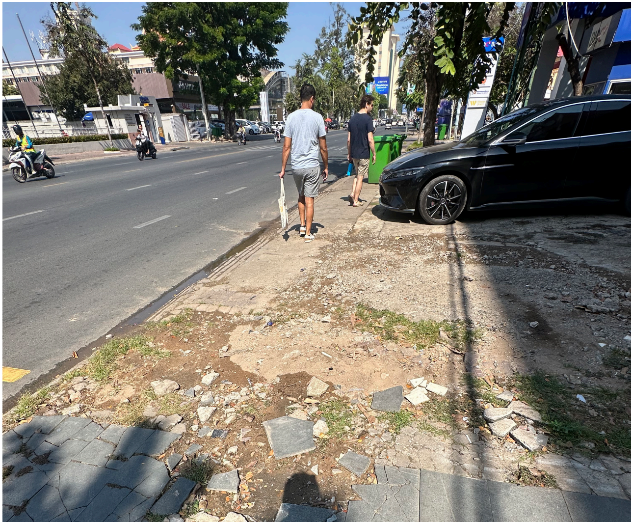
Figure 2. Sidewalk along Monivong Boulevard in Phnom Penh shows damaged sidewalk and pedestrian access blocked by parked vehicles, motorbikes, and storefront activities. (Credit: U.S. DOT Volpe Center)
