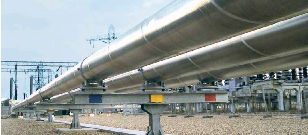
420 kV GIL system at Elstree, London, Great Britain, commissioned in 2004
