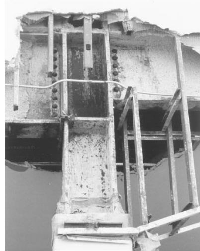
Figure 2. Plastic hinging at top of column (Hall, 1995)
