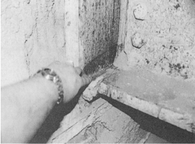
Figure 1. Beam-column connection damage (Kiremedjian, 1999)
