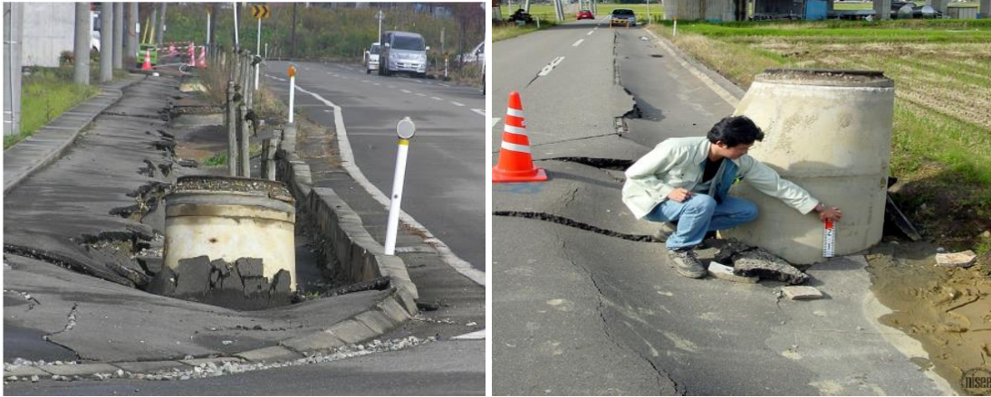
Fig. 4. Flotation of sewage line during the 2004 Chuetsu earthquake (after NISEE 2016).
