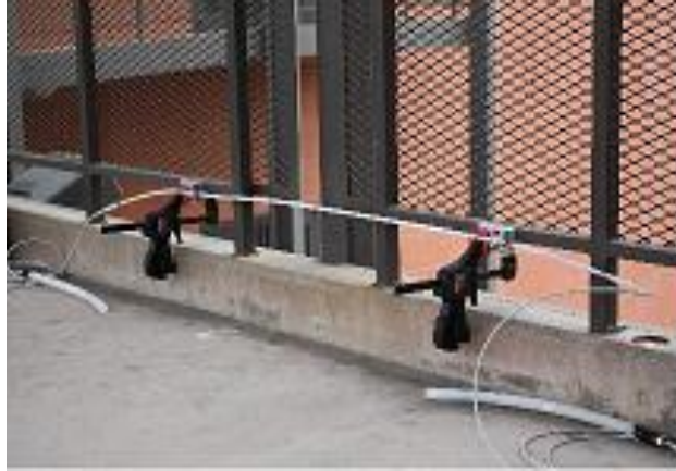
Fig. 11 Fiber optic sensors installed in an overpass for validation test
